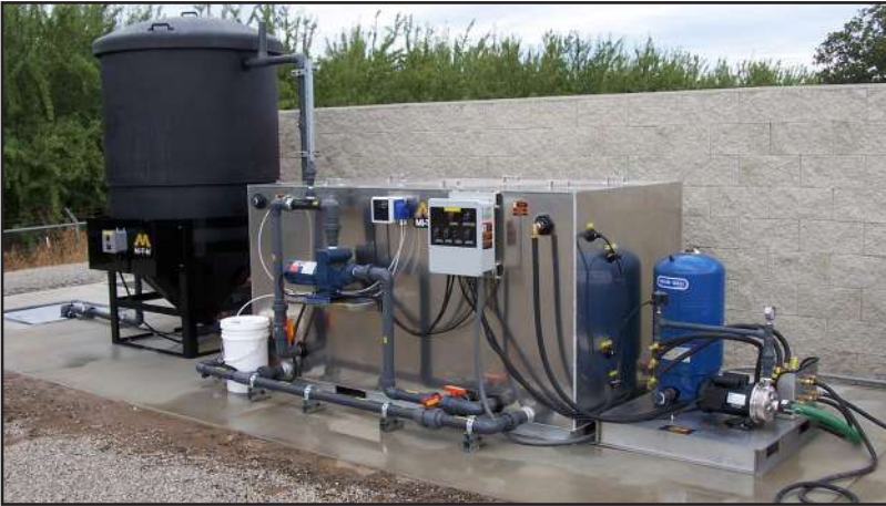
Biological recycle system with WTA Series pretreatment system
