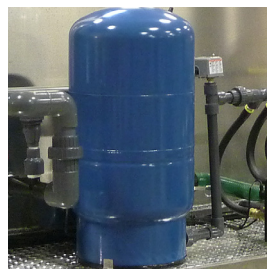
Pressure manifold set-up is standard on BIO-20R-OM11
