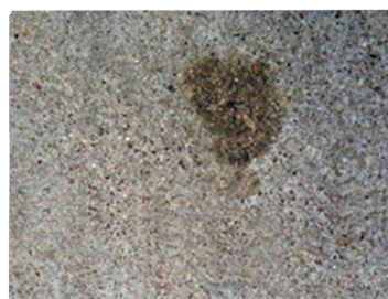
Oil on concrete before treatment
